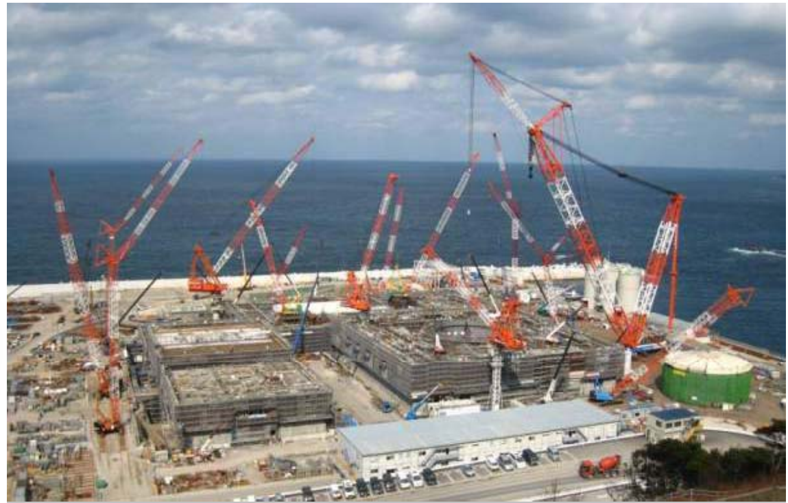
Shimane Nuclear Power Station Unit No. 3 (under construction) The Chugoku Electric Power Co., Inc.
