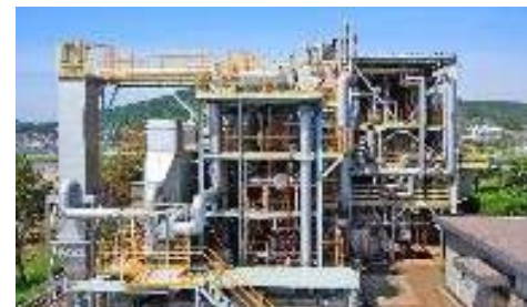
AQCS integrated research facility
